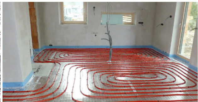
Step 6 - Installation of floor heating After the drying time of at least 48 hours
